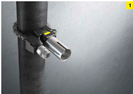
1. Attach a special drill guide on the steel pipe to guide the drilling shaft.
